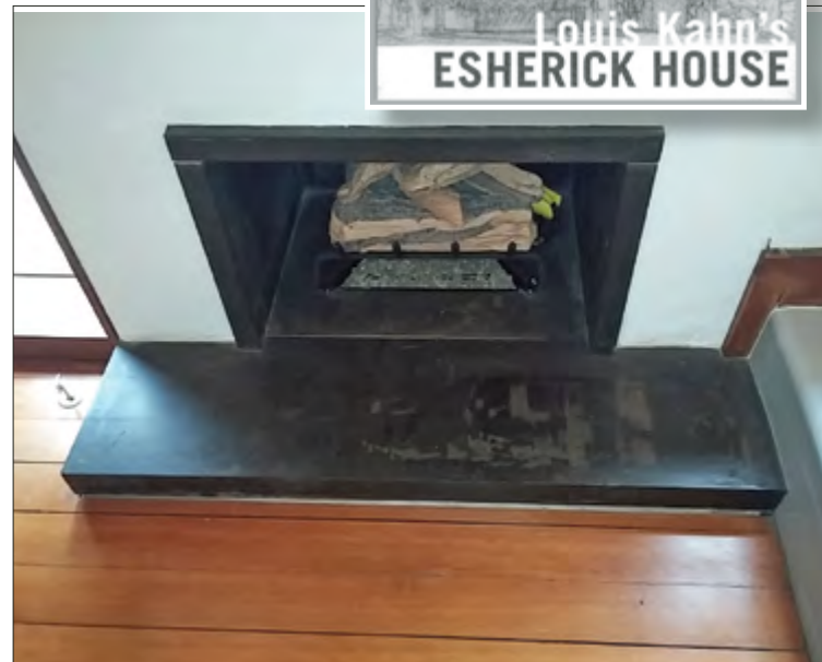
On the soapstone fireplace and hearth restorations: "We did light resurfacing on the hearth, and filled in some voids where the epoxy used back then had cracked and fallen out."
